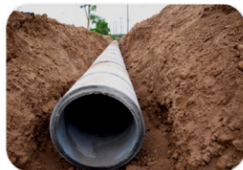
SEWAGE PIPE LINE
