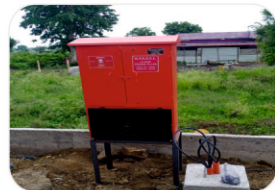
ELECTRIC NETWORK WITH TRANSFORMER
