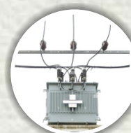
Electric Network with Transformer
